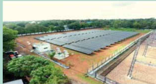
600kWp Solar Power Plant in 110kV Kottiyam Substation
