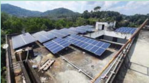
300kWp Solar power plant in Heera college of engineering Nedumangad
