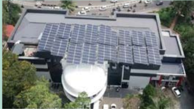
70kWp Solar power plant in District Panchayath Thiruvananthapuram
