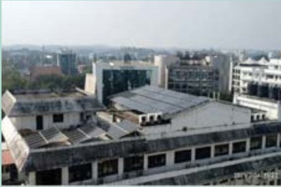
100kWp Solar power plant in Govt. Secretariat
