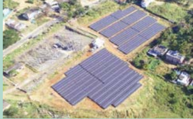
1MWp Solar Power Plant in 33KV Agali Substation
