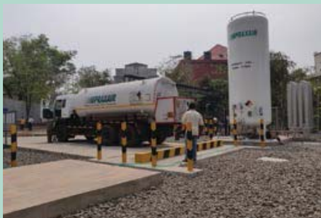
Commissioned Liquid Oxygen Plant at Govt. Medical College Ernakulam
