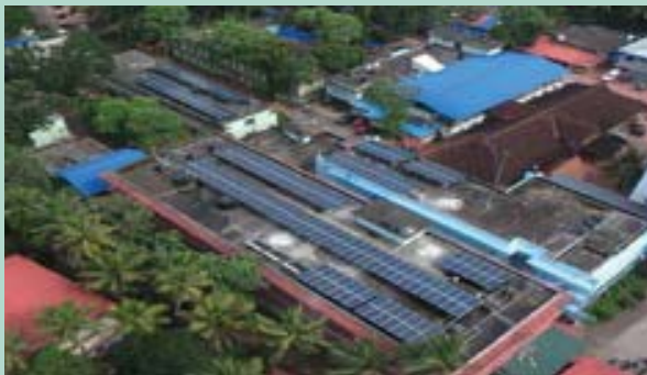
100kWp Solar power plant in General hospital Neyyattinkara
