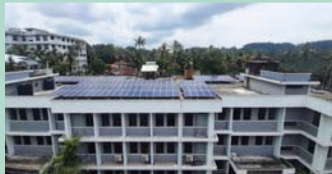
300kWp Solar Power Plant in Mohandas College of Engineering
