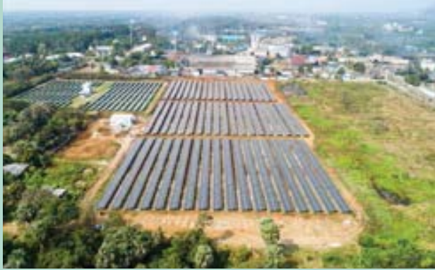
3MWp Solar Power Plant in 220KV Kanjikode Substation
